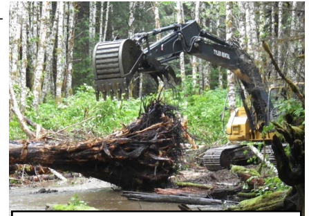
2014: placing large wood in Saginaw Creek to restore stream function and habitat features.
